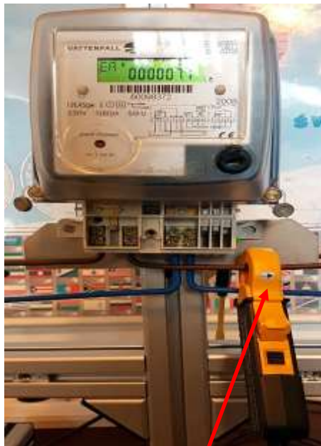
Current clamp closed on phase to load cable. Note direction =>!
